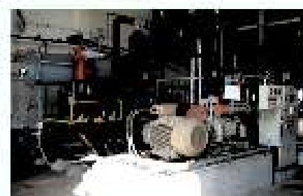
Brine plant (-25°C)
