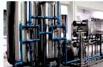
Water Purification System
